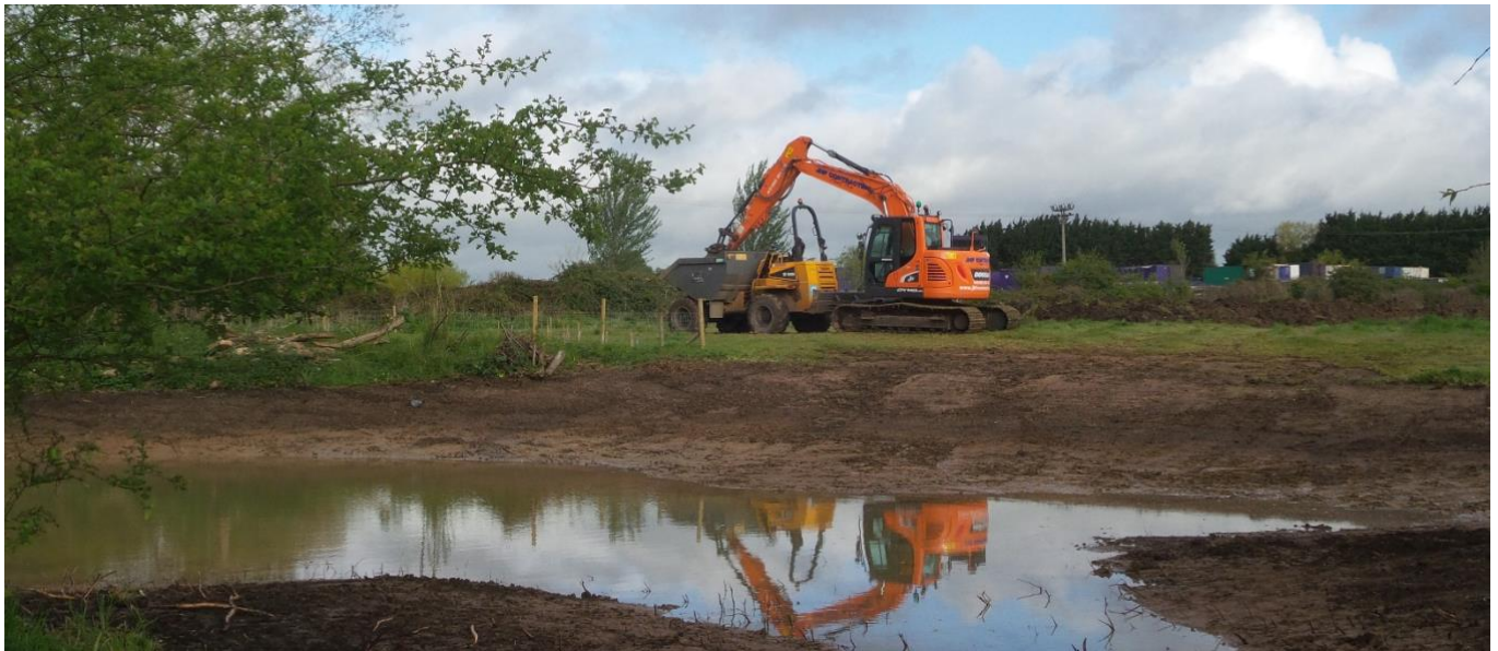
02. Work underway to resurrect the ghost pond at Mill Bank Meadows, Fladbury 10.05.21. Gary Farmer.
